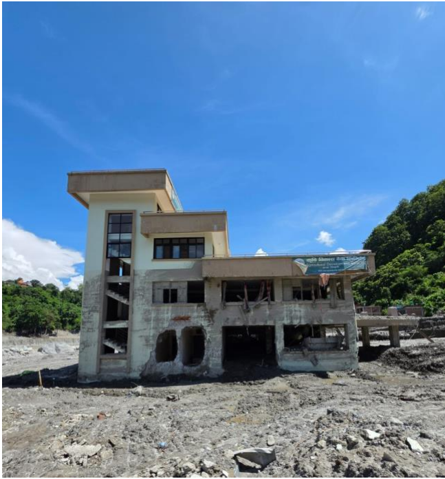
The Agricultural Development Bank — lower floors destroyed, upper structure still standing, signage still legible.
